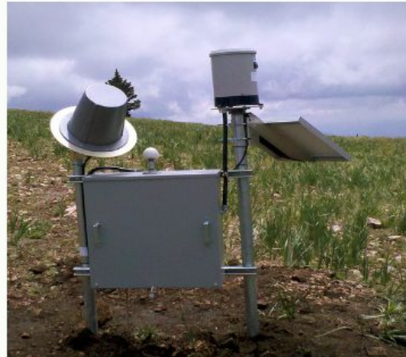
A precipitation gage with solar panel, radio stand, and electronics installed within the burned area of the Whitewater Baldy Complex Fire, New Mexico (Photo: Kristen Lemoine, NRCS New Mexico)
